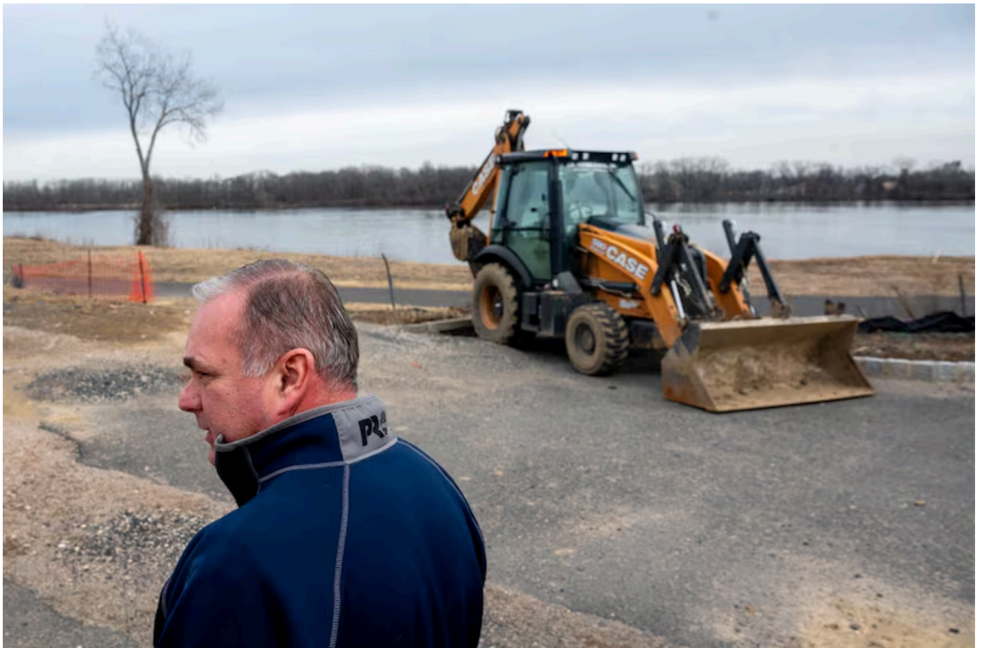
Builder Bernie Sauer along the Delaware River at his under-construction Radcliffe Court on the Delaware.
